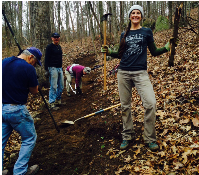
Chattanooga Hiking Club members help with the reroute of the top section of the trail.
